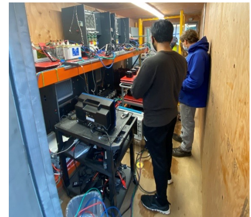
Demonstration of the entire MUSE-SST system in the mobile container
